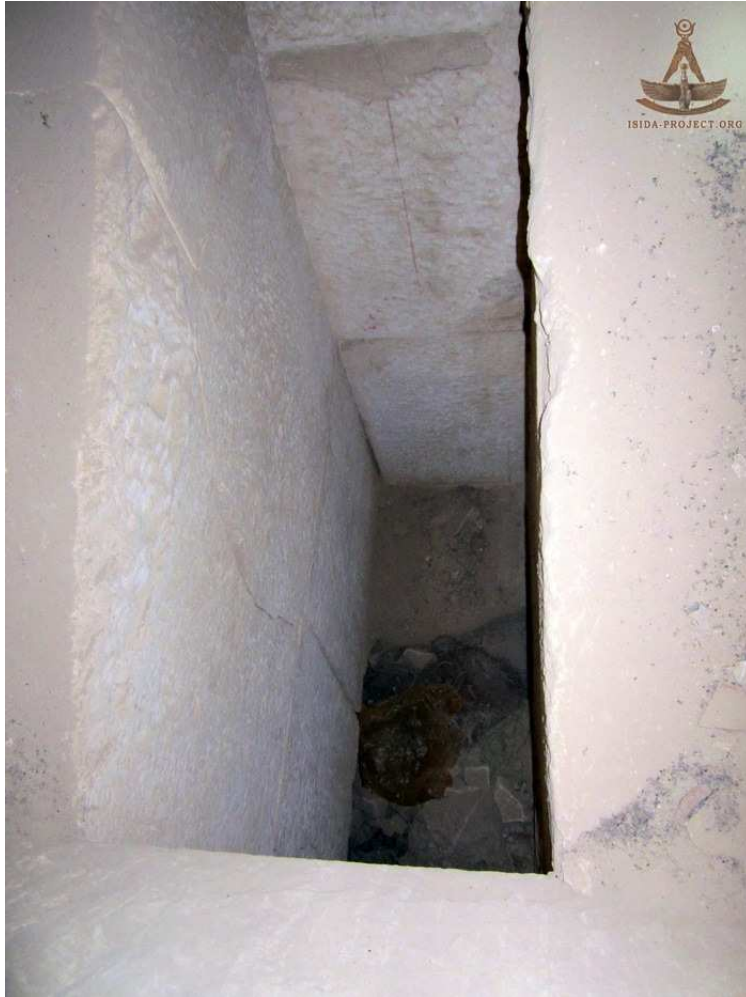
Looking down into the pit, a faint red line denoting axis can be seen on one of the blocks.
