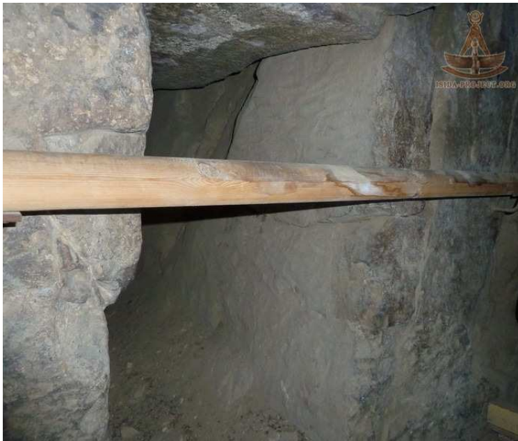
A view into the excavated east wall showing the face of the continuous joint.
