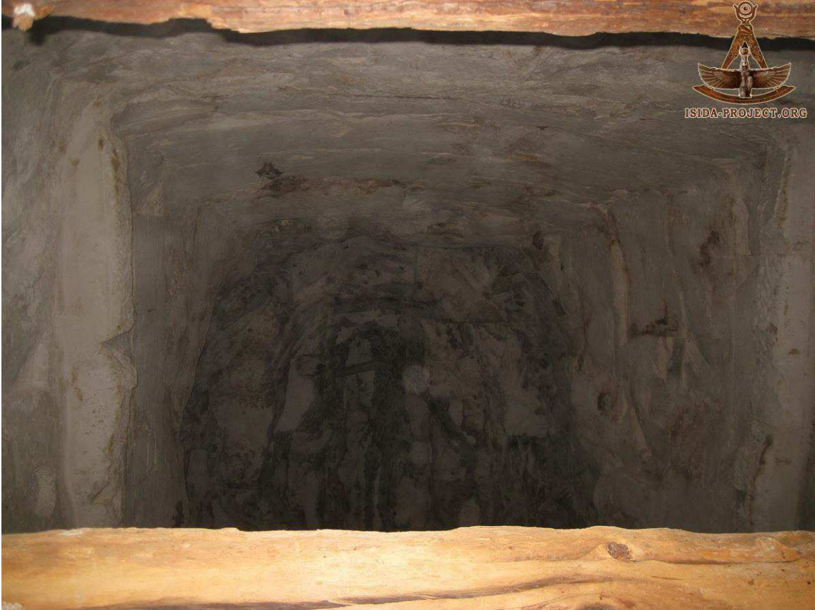
Looking through the beams at the damaged ceiling.
