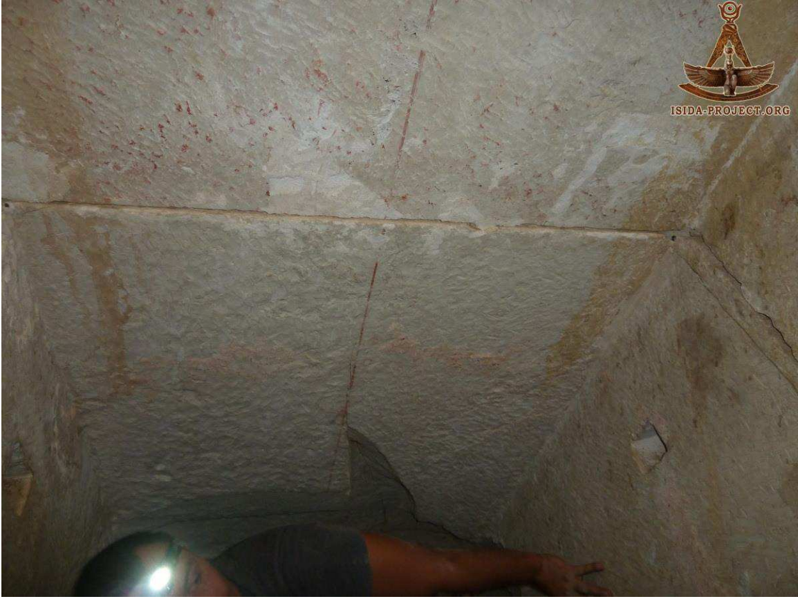
The continuous joint running along the ceiling, note red line defining axis of passage.
