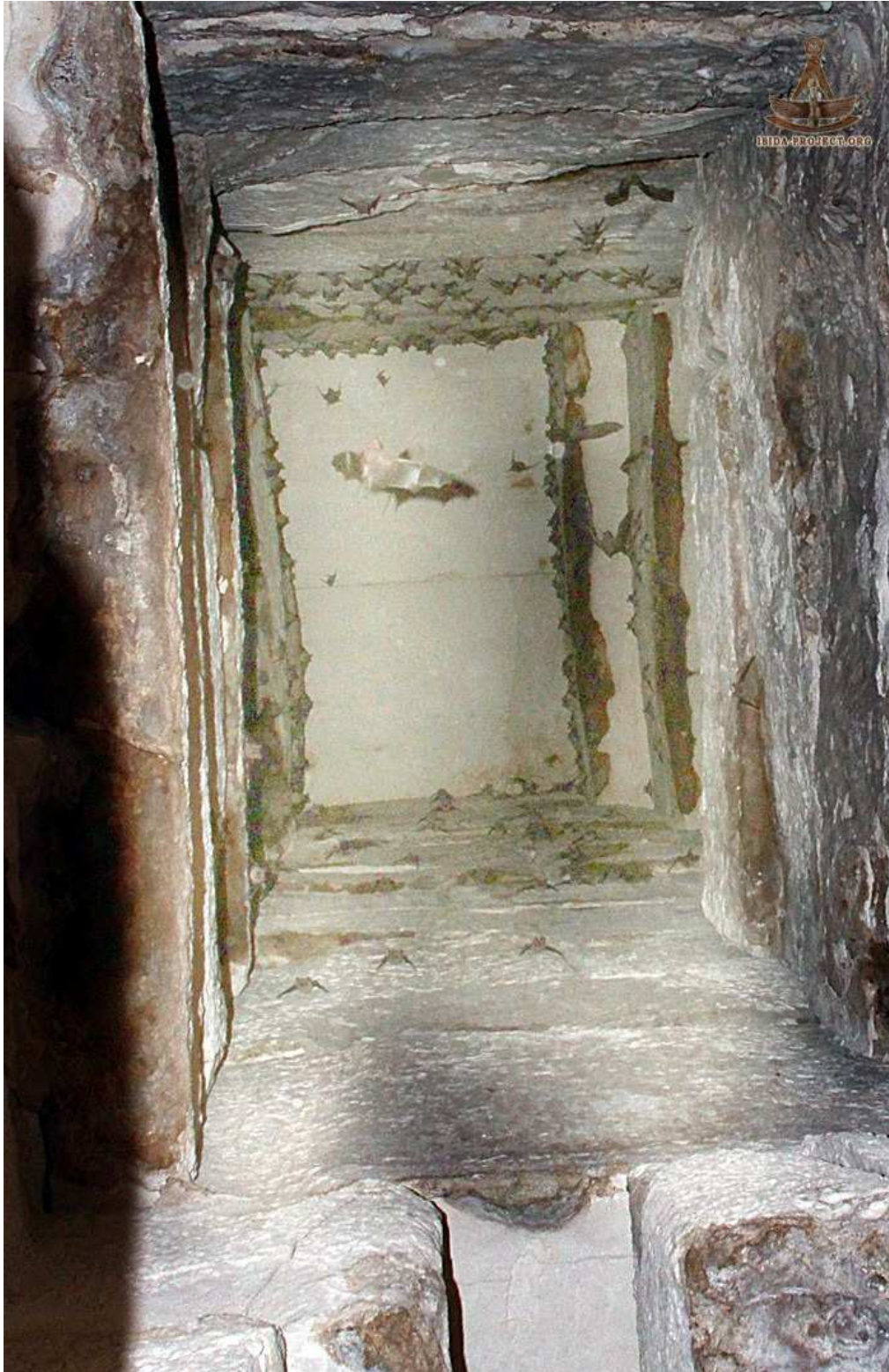
The top of the chimney, here we see the join between the two stones that close the top of the chimney.
