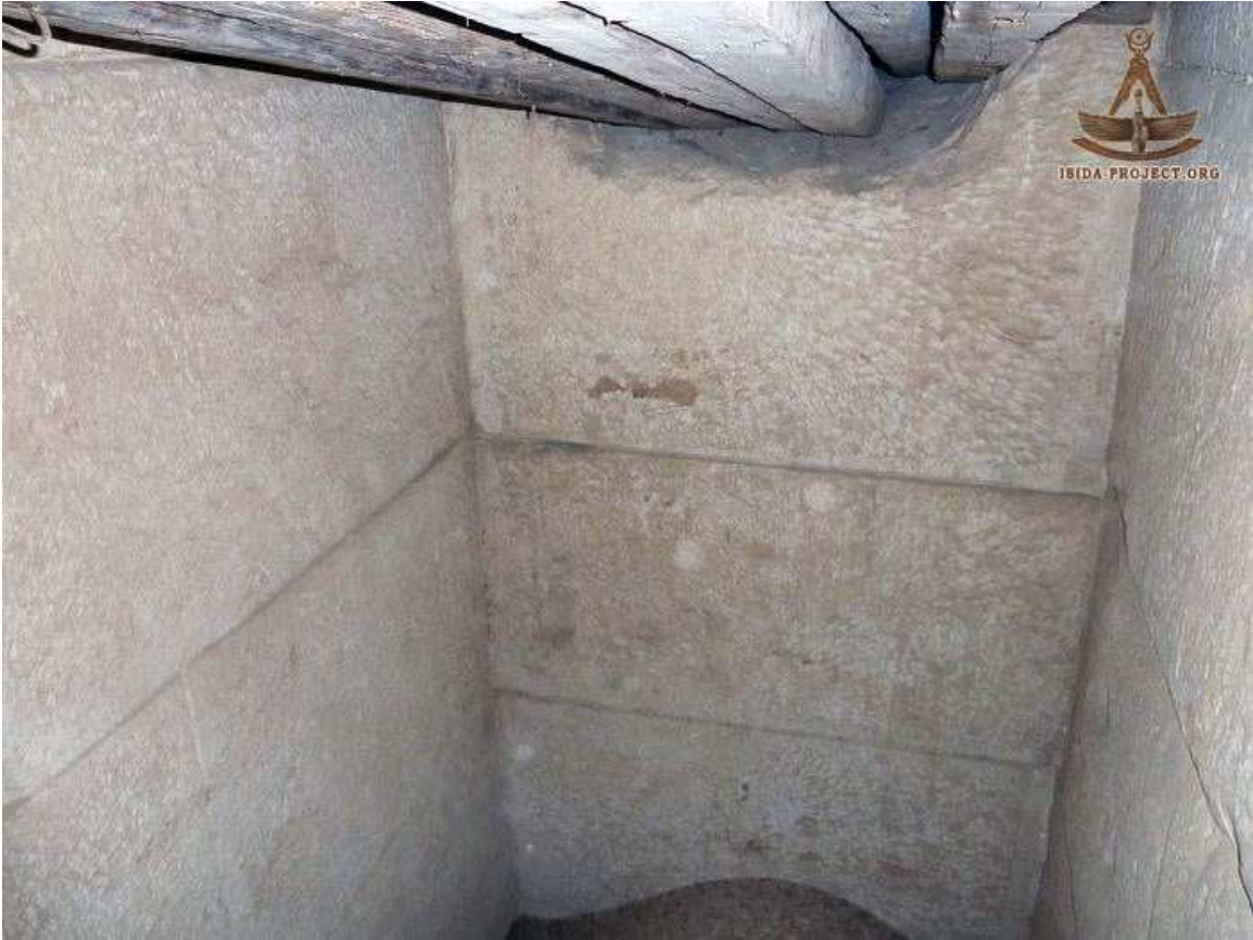
Looking at the west wall of the shaft with its top edge rounded.
