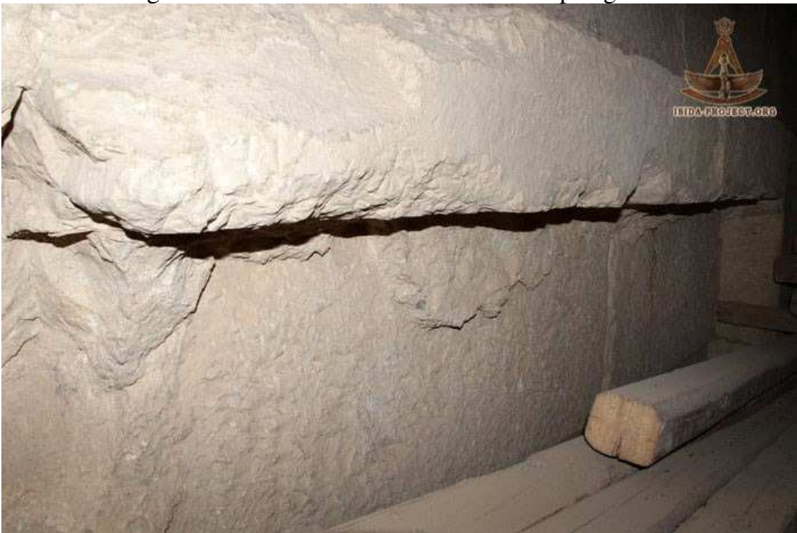
The width of the shaft undercuts the walls.
