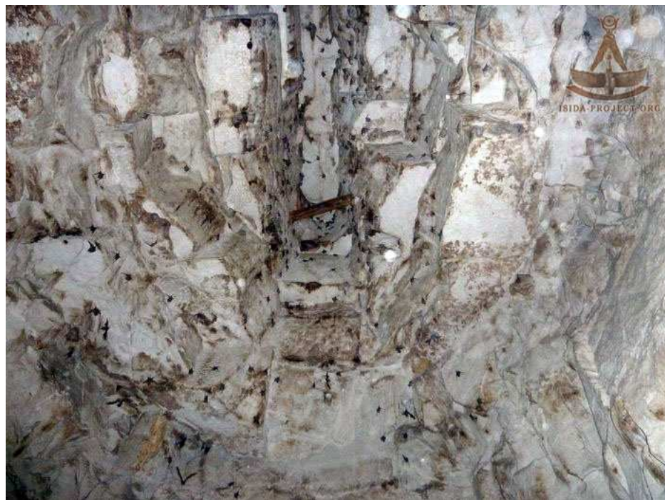
The damage is quite extensive
