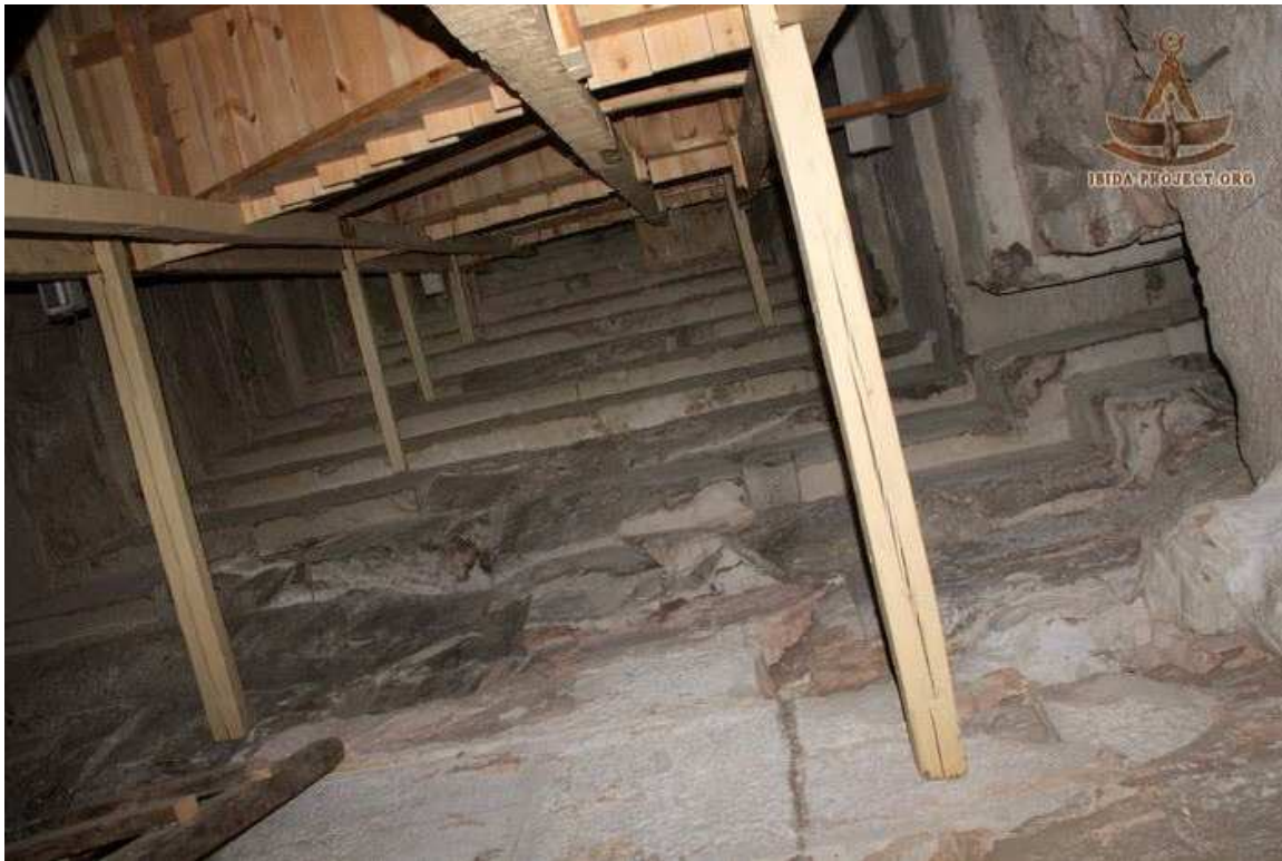
Looking up at the ceiling along the east wall, the entrance into the corbelled window can be seen on the right.
