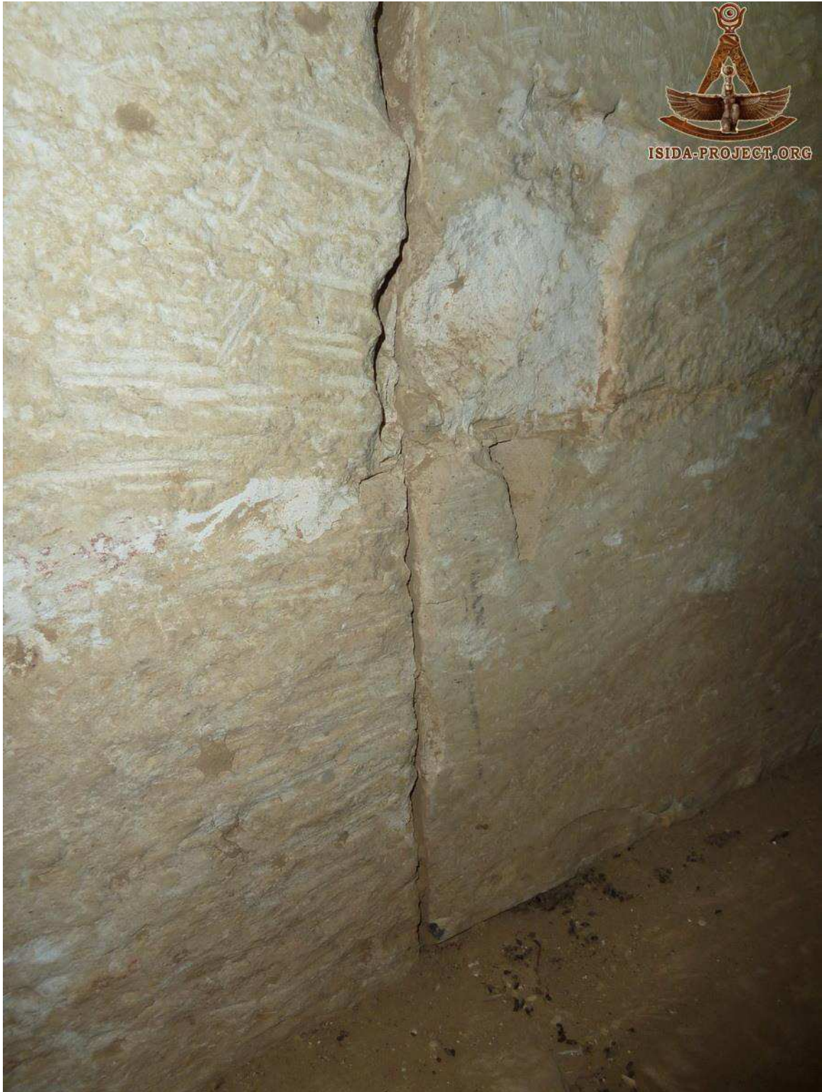
The continuous joint on north wall of west passage.
