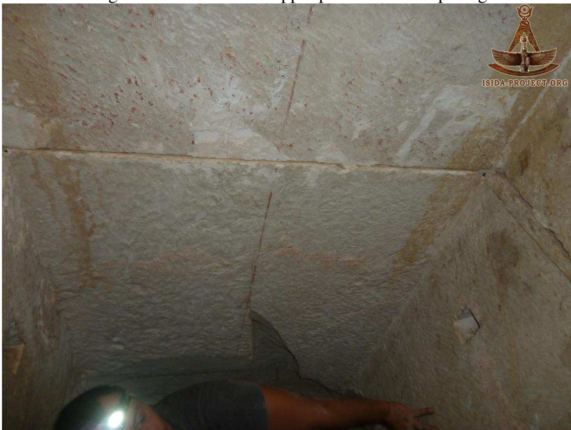
West passage continuous joint, here we see the ceiling joint meet the joint on the south wall. Also note the small square hole and red ochre line.
