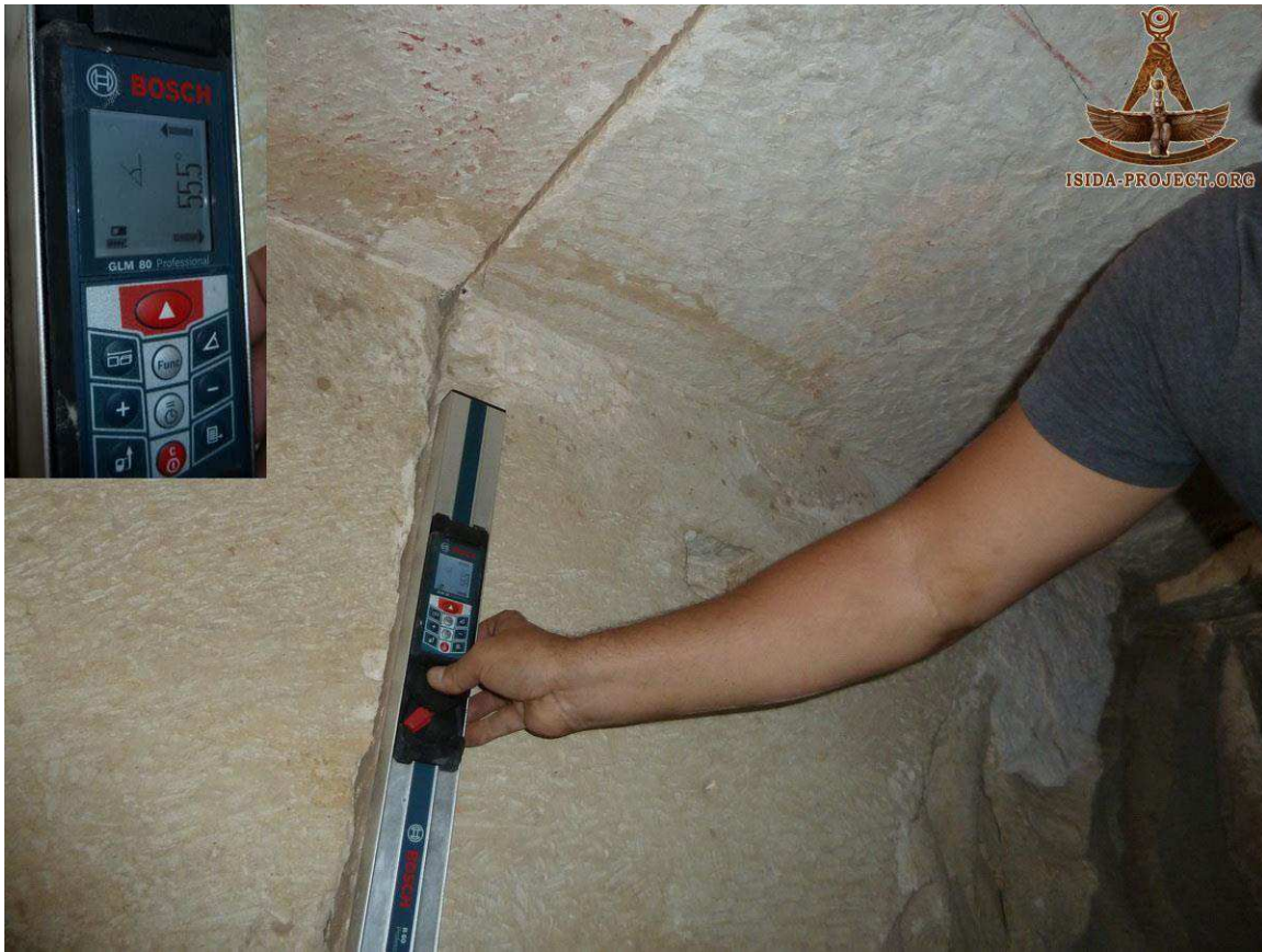
View of the continuous joint in the western passage measuring 55.5 degrees, north wall.
