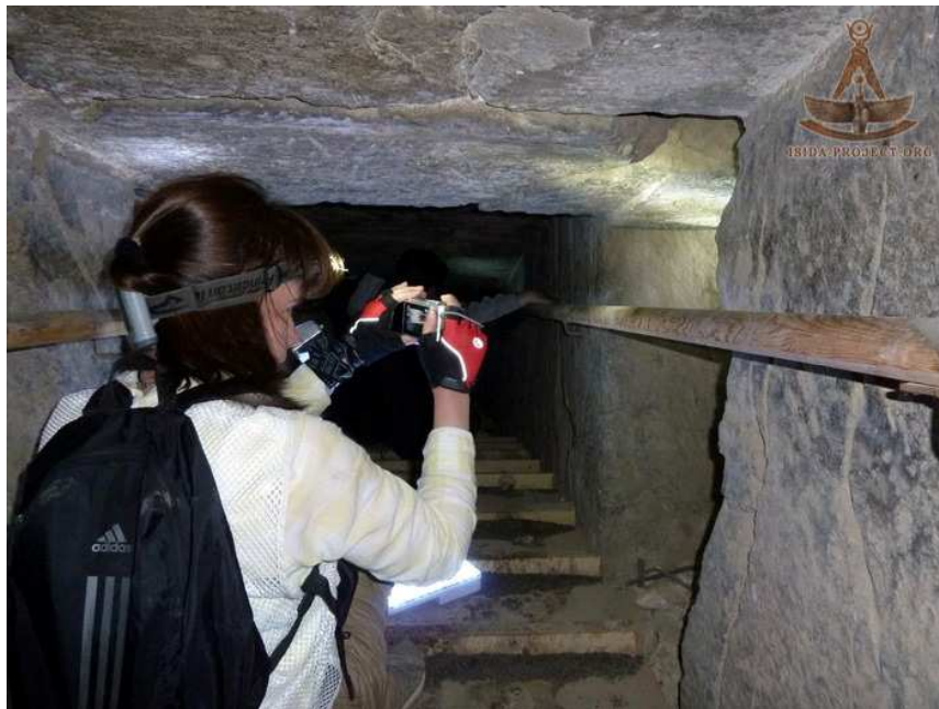
Looking down the northern passage at the continuous joint. The wall blocks immediately north of the joint have been excavated sometime in the pyramids history; the western wall block has been excavated up to 2m deep and .85m wide, the eastern wall block has been excavated to a depth of 1.1m and .75m wide.
