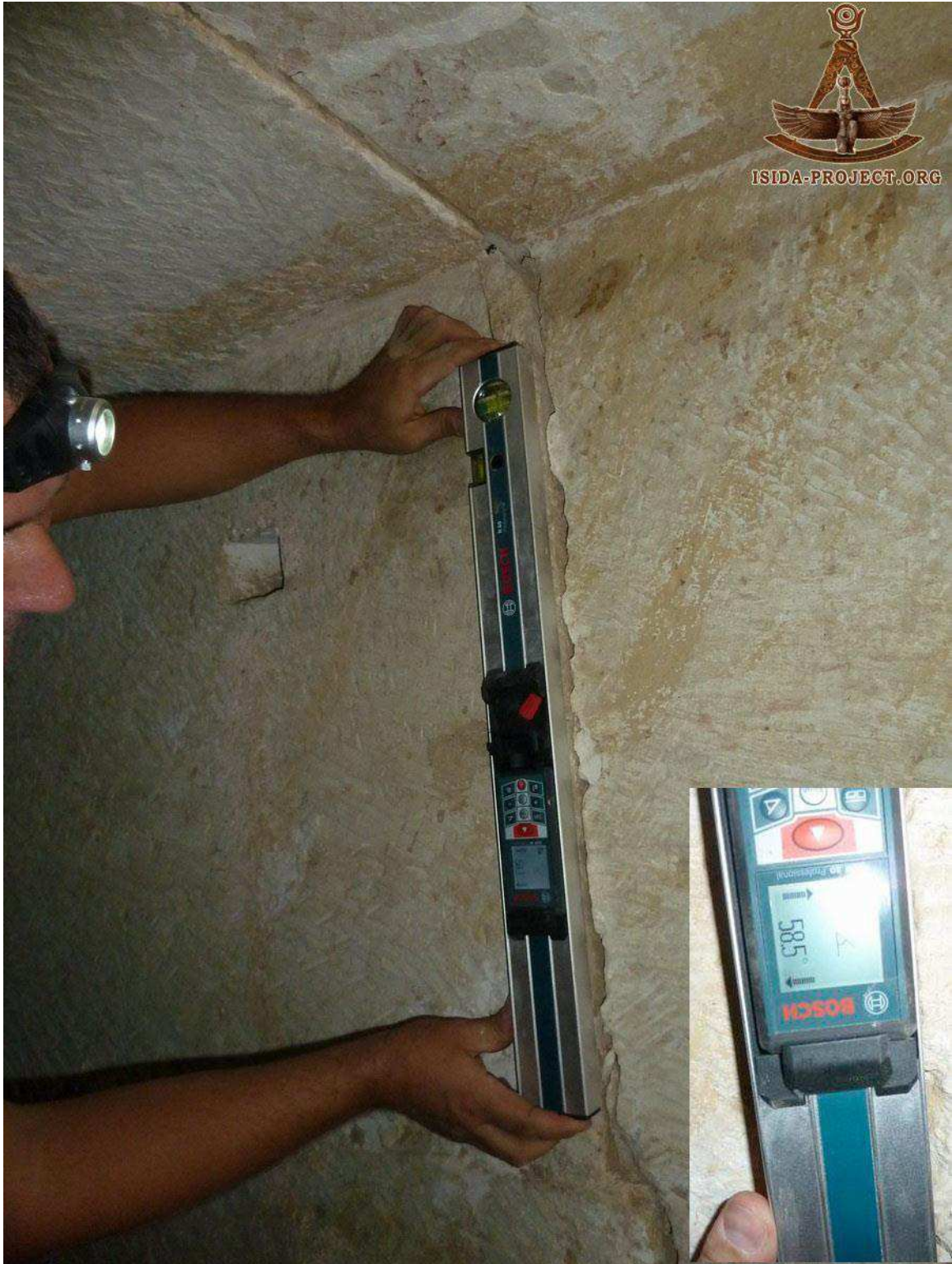
View of the continuous joint in the western passage measuring 58.5 degrees, South wall. Note also the square hole in the wall.
