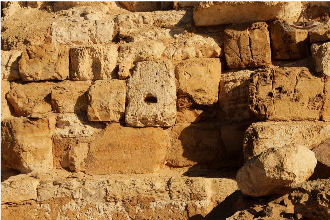
Close up view of core masonry, traces of pink mortar still visible
