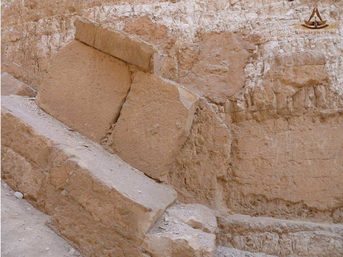
Another view of surviving cladding stones on east wall, patches of pink mortar can be seen adhering to the trench walls.
