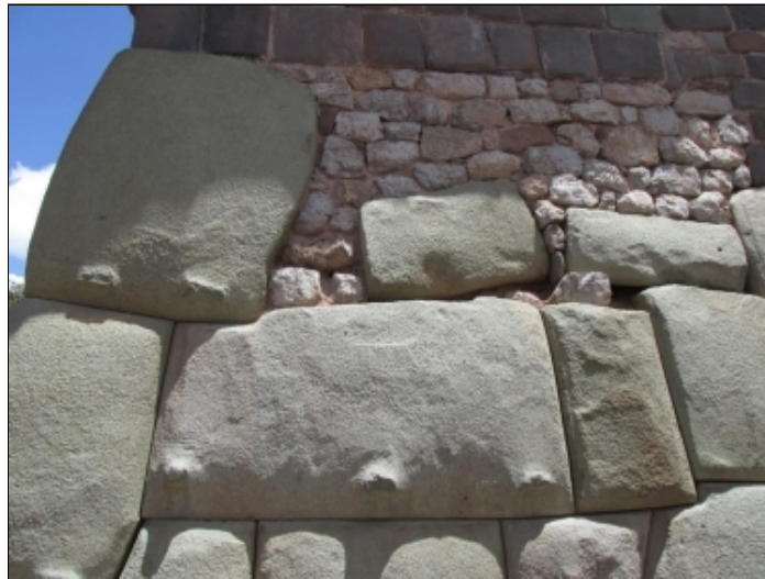
Inca Roca wall showing inferior repairs above
