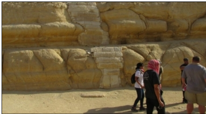
Signs of extreme weathering in the Sphinx enclosure
