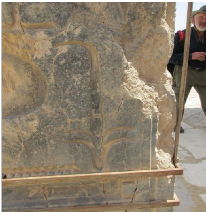
Portion of the remains of the right gate with seeming internal crystal expansion
