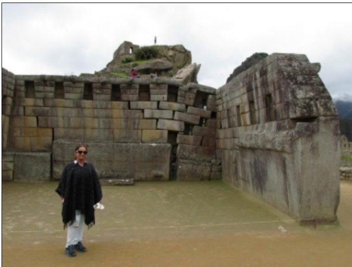
Wall showing extreme catastrophic damage
