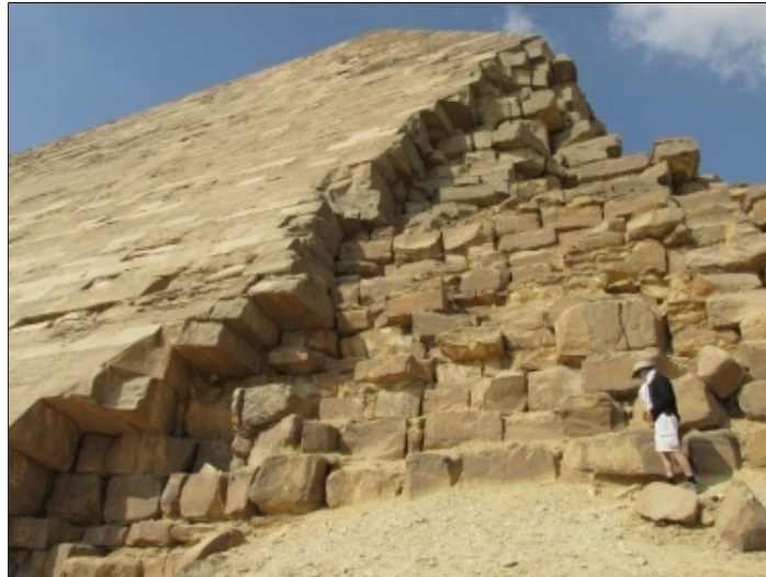
Photo of damage to one of the four corners of the Bent Pyramid
