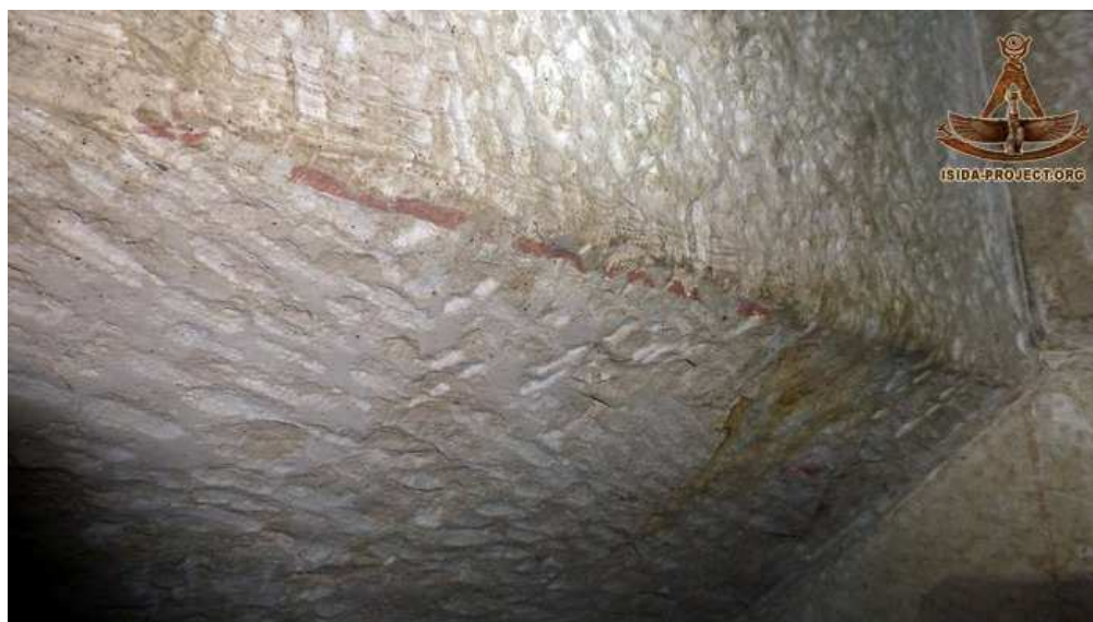
Red guide lines visible over top edge of chamber doorway and a vertical line running down the east wall
