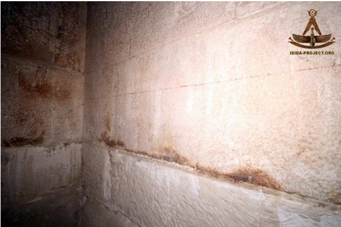
Level line along west wall and missing flooring
